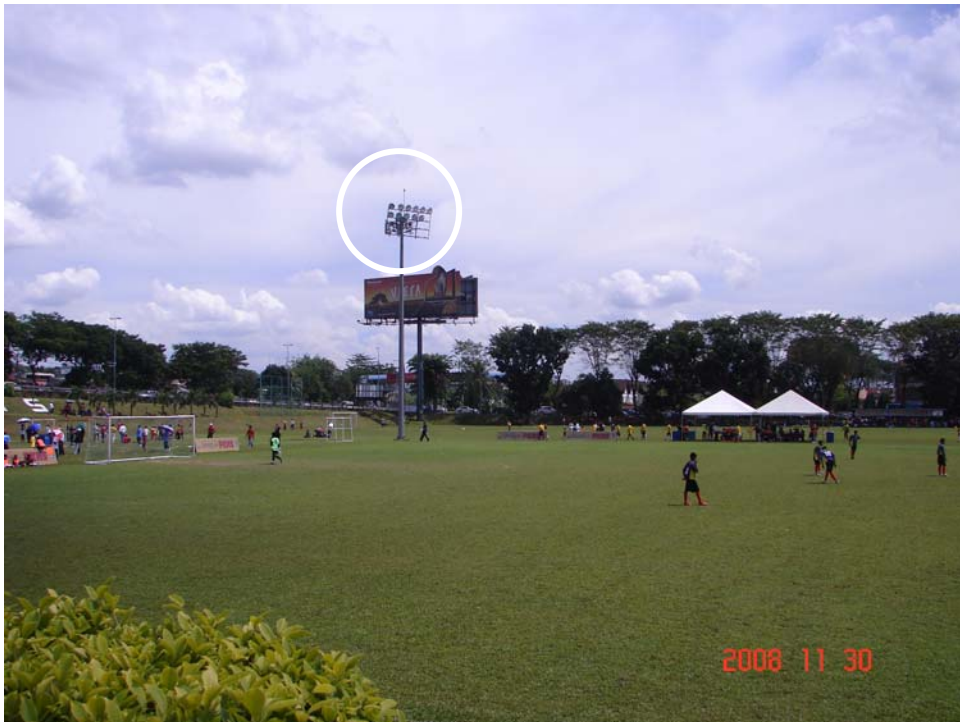
Fig. 15: An ESE lightning rod installed on the floodlight of a football field.
