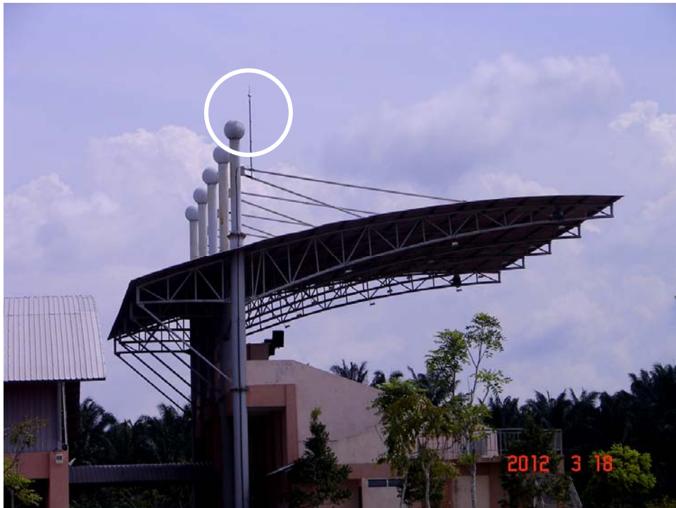
Fig. 5: The Satelit ESE lightning rod mounted on the metal pole.
