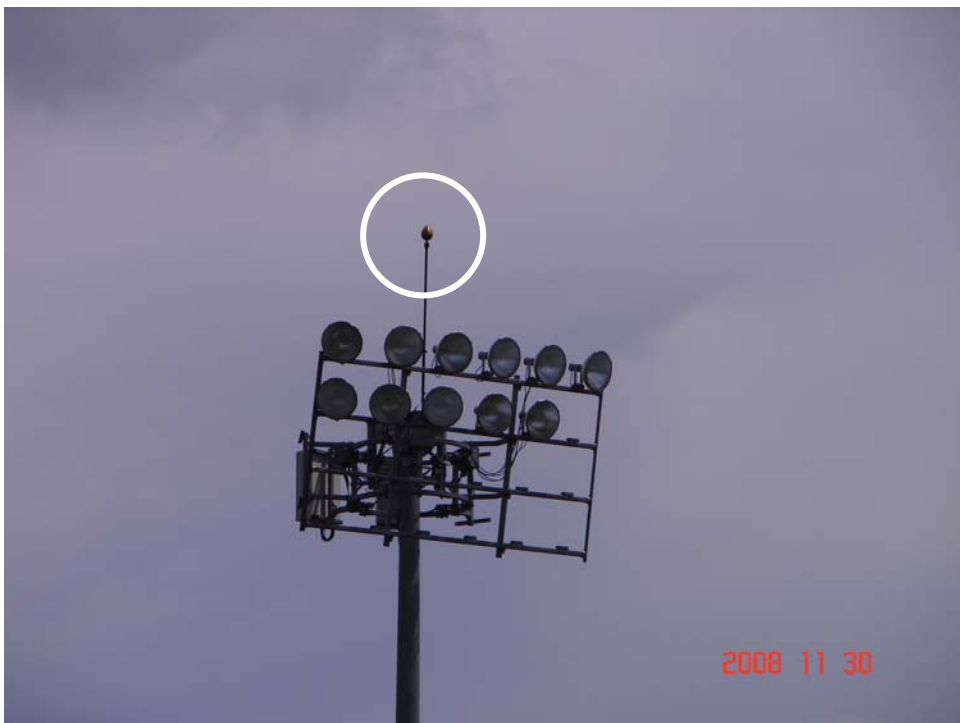
Fig. 16: A close-up photograph of the ESE lightning rod.
