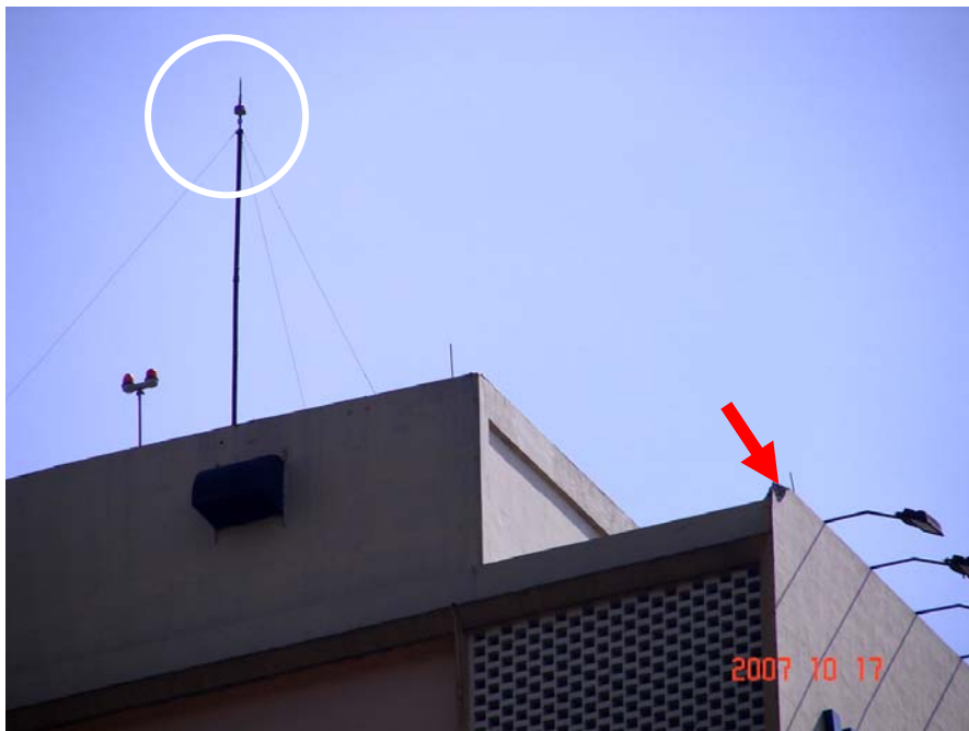
Fig. 12: The Wisma Tanah building in 2007 (before the damage was repaired).
