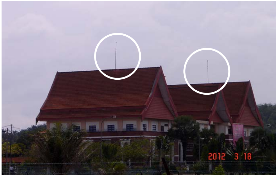
Fig. 1: KUIM administrative building with the ESE lightning rods.
