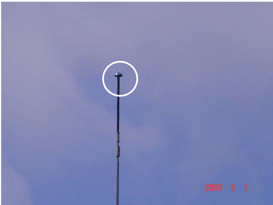
Fig. 14: A close-up photograph of the ESE lightning rod.
